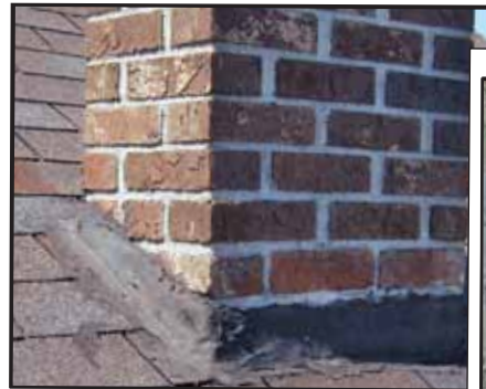
Chimney with cracked and deteriorated flashing
